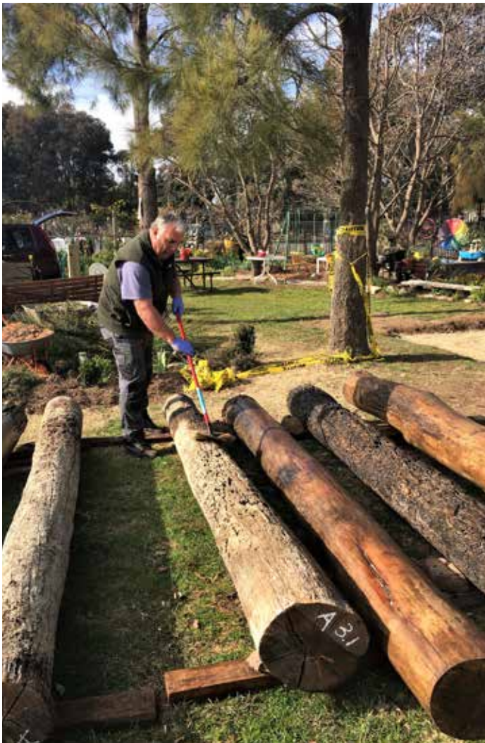
Bill Ashley oiling the massive pole supports for the garden shelter. Some of the poles came from the Bateman's Bay wharf and have intricate surface textures
