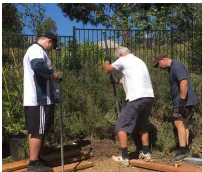
Stephen, Alan and Joe using a crowbar on the final hole, solid rock – score: hole 1, men nil. A jackhammer was finally successful.
