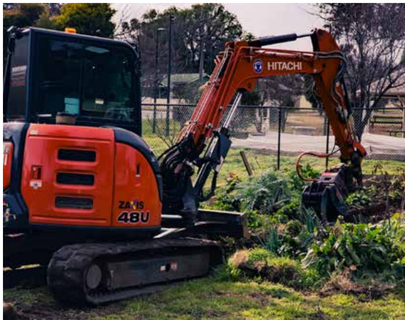
(above) The big guns engaged; (below left) extracting buried rebar; (below right) one of several loads of metal edging headed for recycling. Photos: Elisa Pevere
