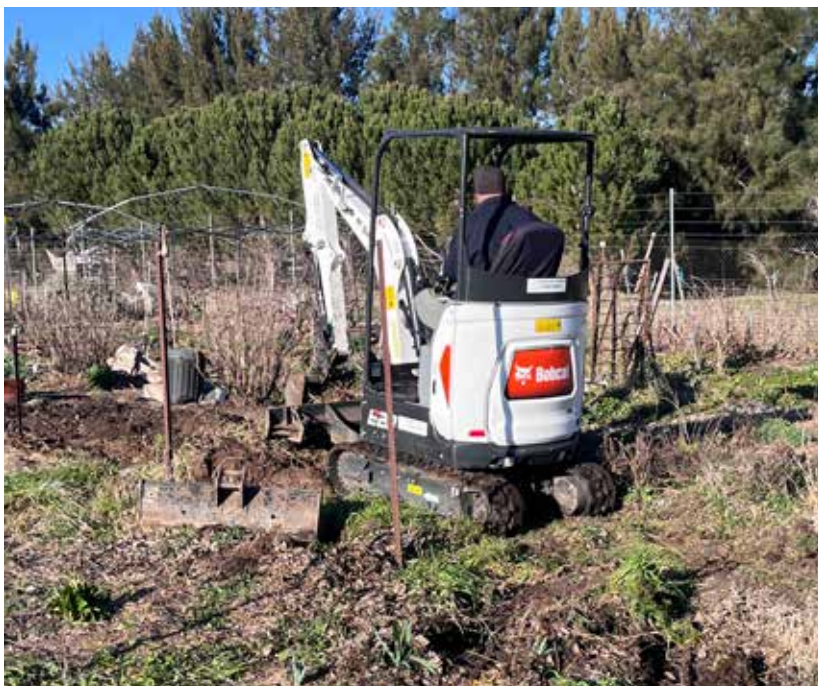
Hiring a digger is a good way to quickly accomplish jobs that even many hands would take a long time to do. Old and unproductive fruit trees were removed to make way for an orchard refurb. (Photo: Lisa Walkington)
