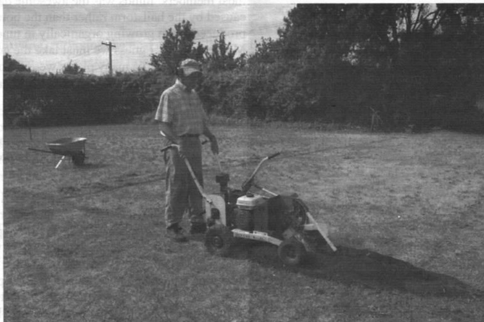
Alan Robertson turns the first sod—for the water pipes at O'Connor community garden
